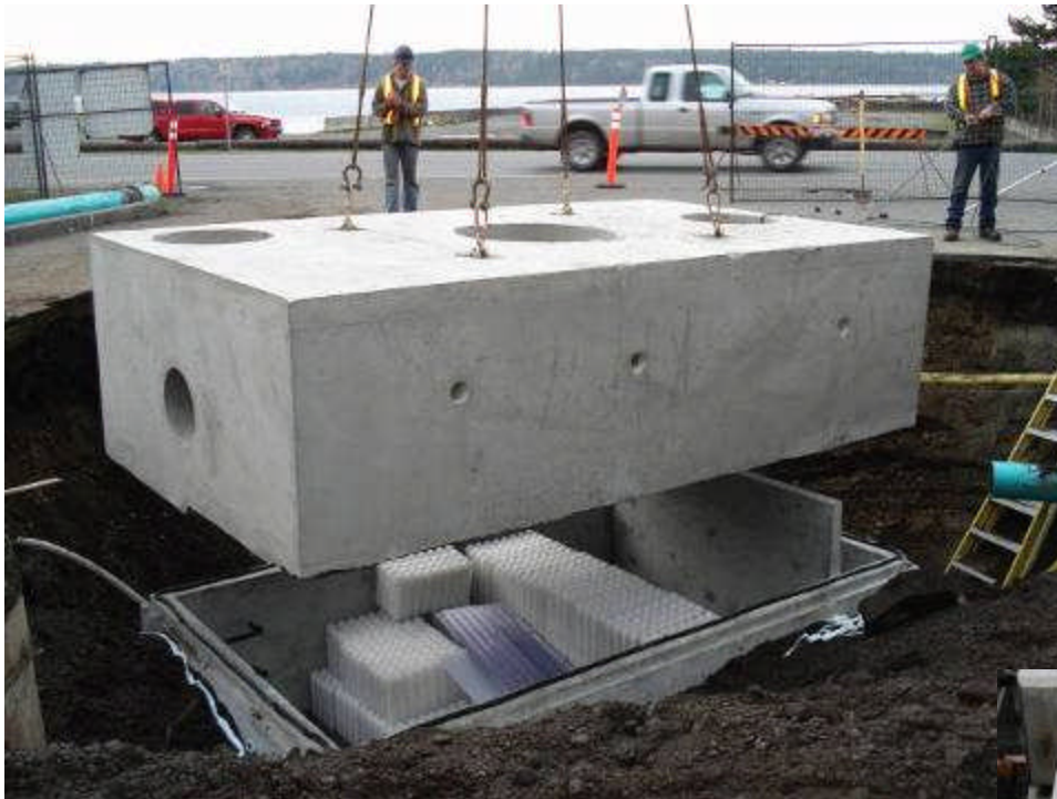
Field-Assembled Precast Vault at Service Station
